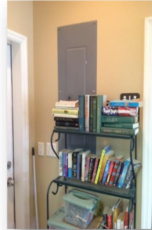
An example of a violation; Blocking access to the electrical panel.
